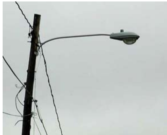
Cobra lighting may be appropriate where large areas need to be lit. However, this lighting can be intrusive to nearby residents.
